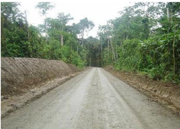
Figure 21. A completed portion of the Petrobras road to the boundary of Yasuní National Park, June 2005. (Photo courtesy Save America's Forests )
